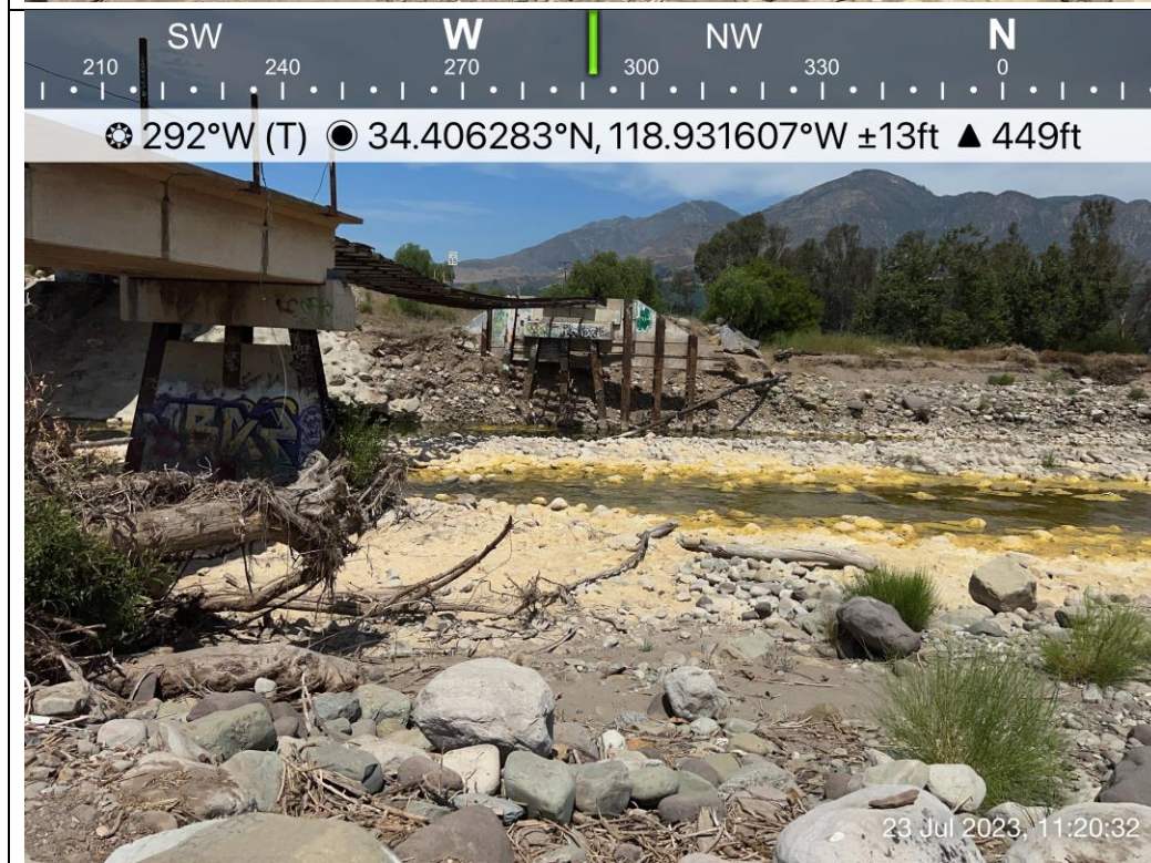
Photo 6. View of damaged bridge looking northerly.
