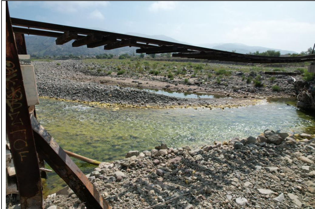
Photo 1. View from damaged abutment looking east
