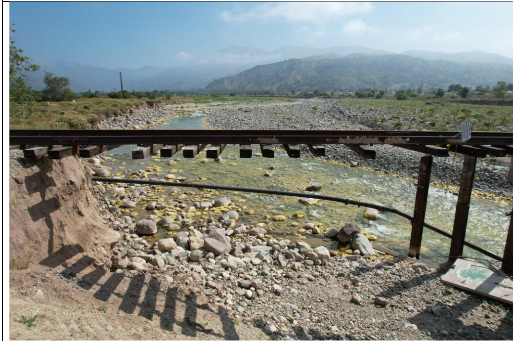
Photo 2. View of 2024 storm damage. Looking East
