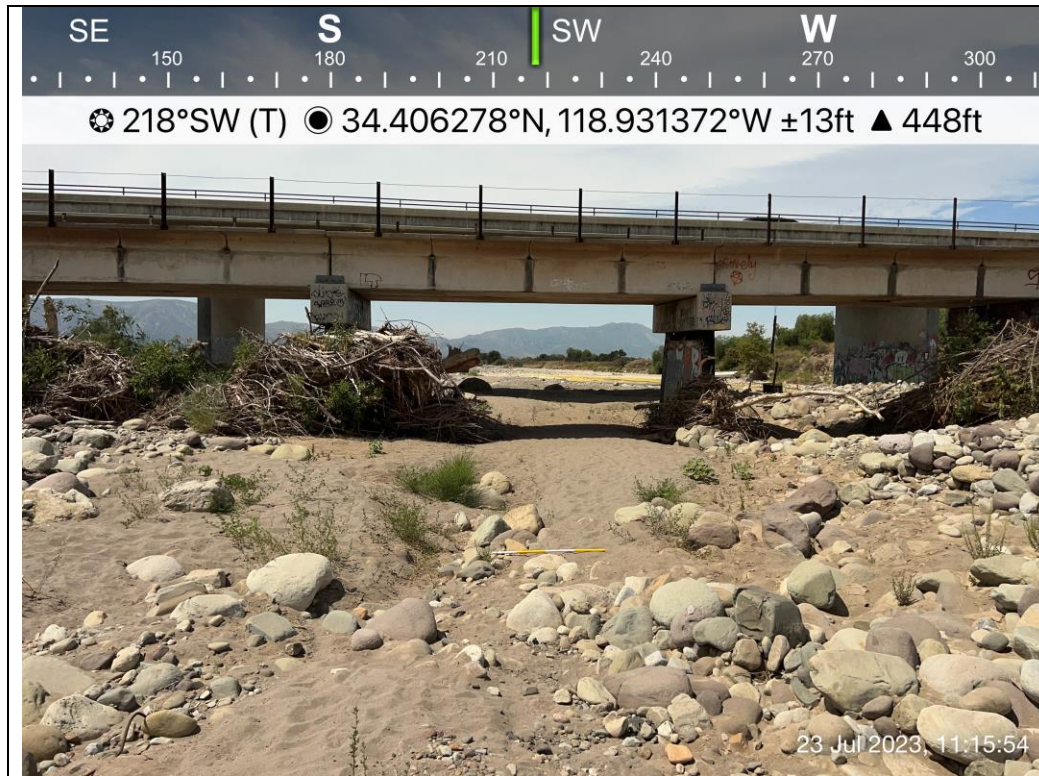
Photo 5. View of debris on undamaged section of the bridge. Looking West
